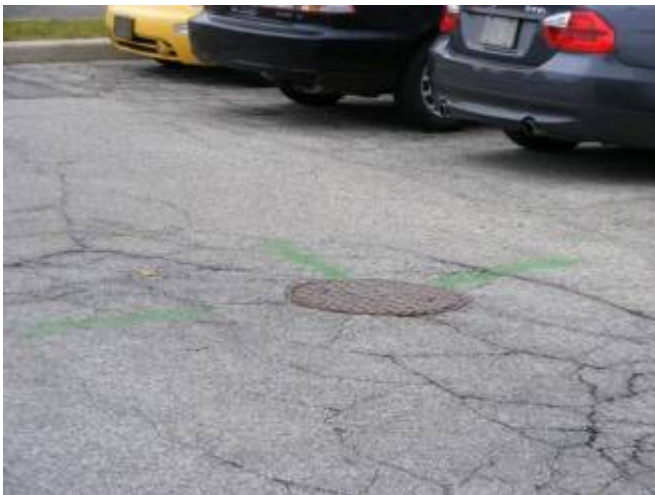
Cracking, upheaval, potholes (saturated granular bases, inadequate base, poor drainage)
