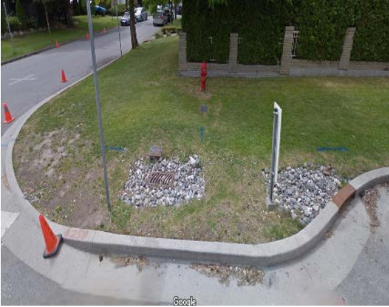
Design lacking in stormwater function
