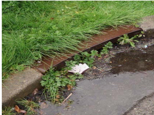
Inlet clogging, requires re-design of pre-treatment
