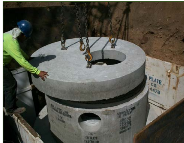
Oil and Grit Separator
