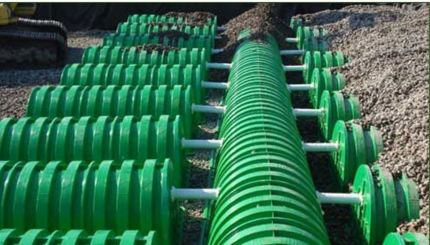
Underground storage and pretreatment
