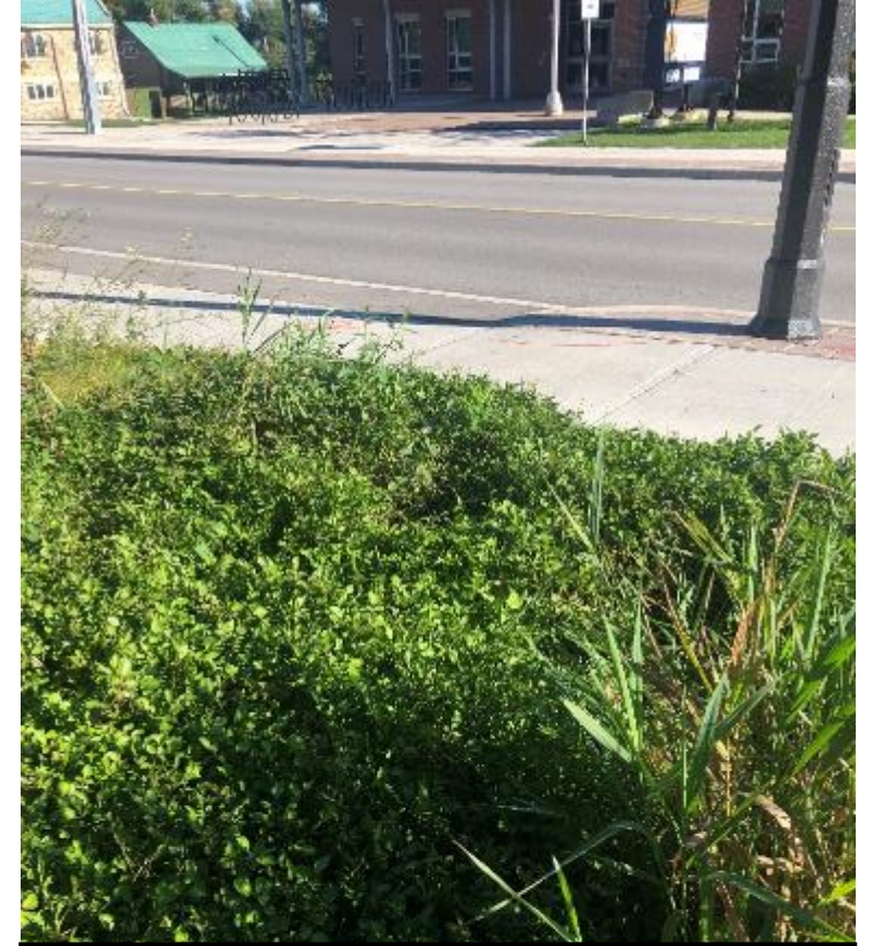
Catchbasin choked with watercress
