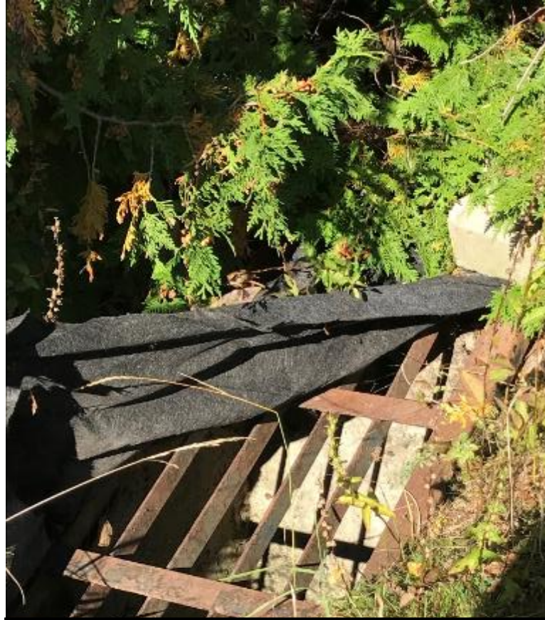
Catchbasin covered with filter fabric
