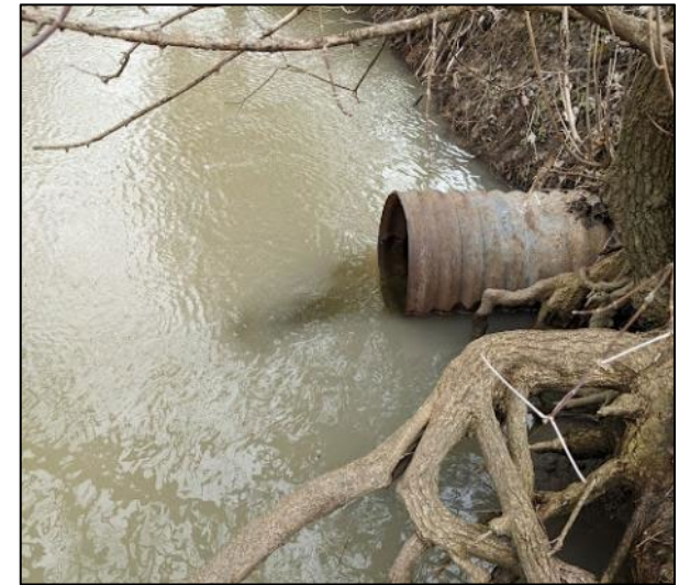
Stormwater drainpipe located at site SWM04
