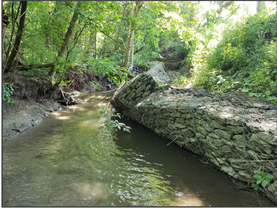
Slumping Failure Of Gabion Baskets
