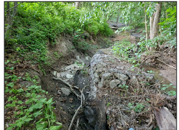
Flow Restriction Posed by Failed Gabion Baskets
