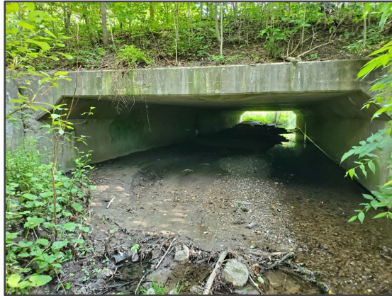
Accumulation of Sediment in Culvert
