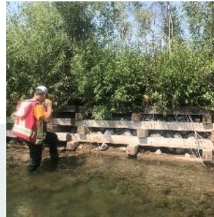
VEGETATED CRIB WALL Sample size: 10
