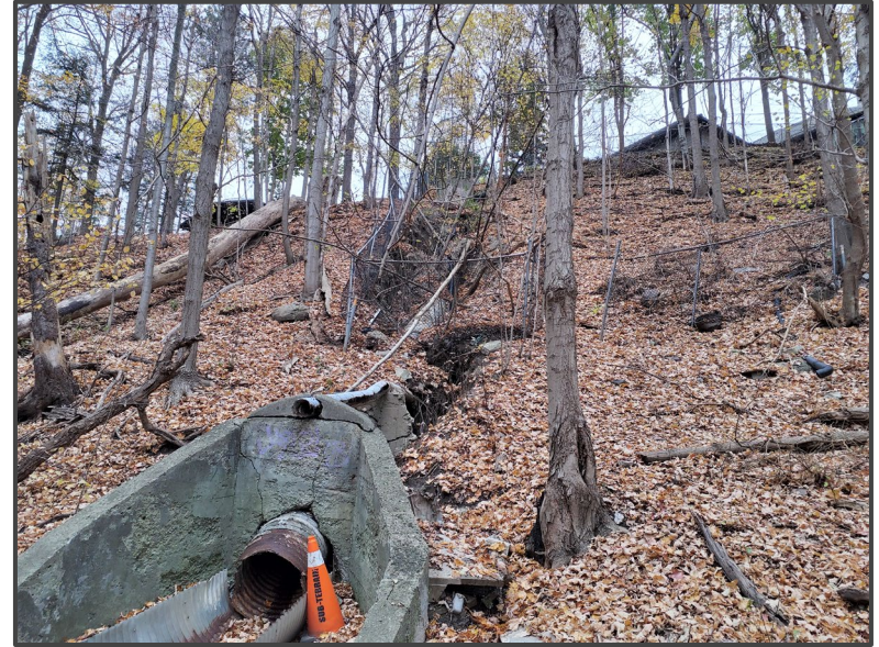
Erosion Gully Formation Along Valley Slope
