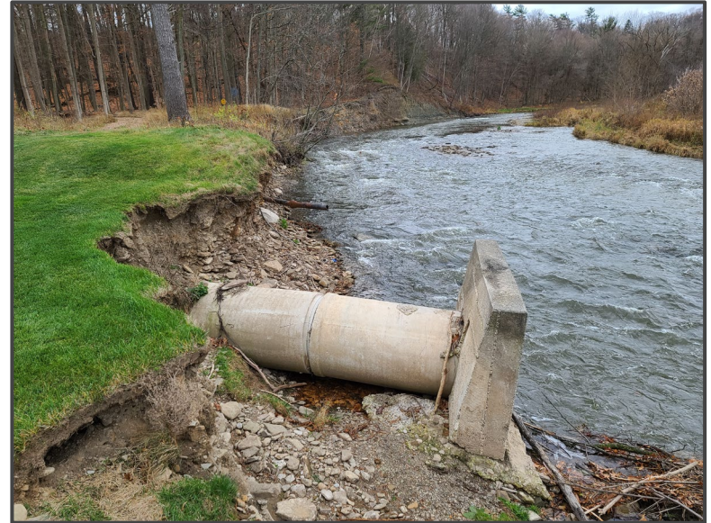
Outflanked Headwall Structure and Upstream Pipe Segment
