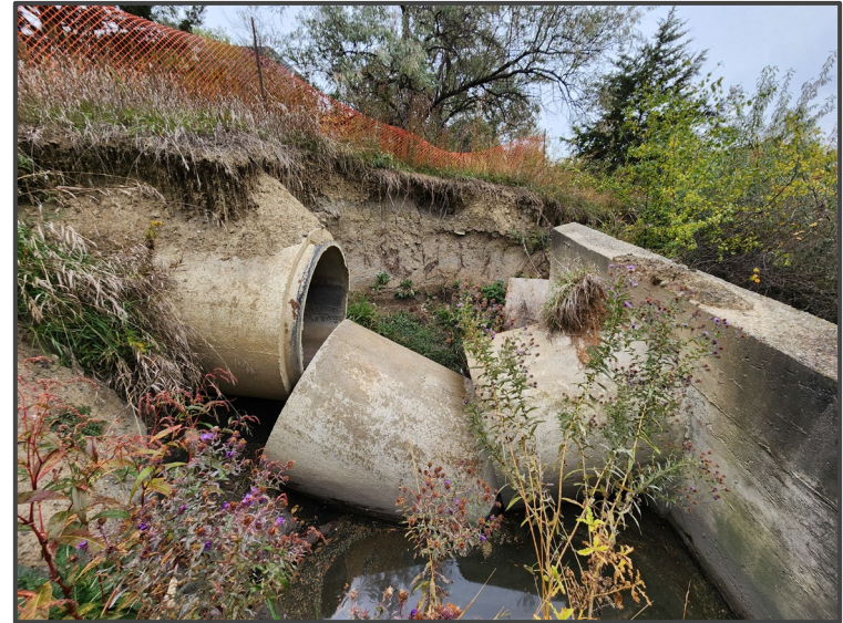
Collapsed Concrete Headwall Structure and Failed Upstream Pipe Segments
