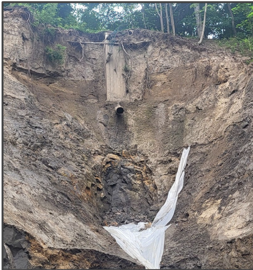
Manhole at Imminent Risk of Failure
