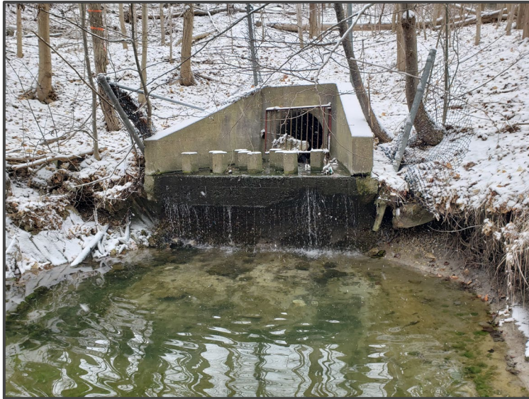
Undermined Stormwater Headwall Structure at Risk of Collapse
