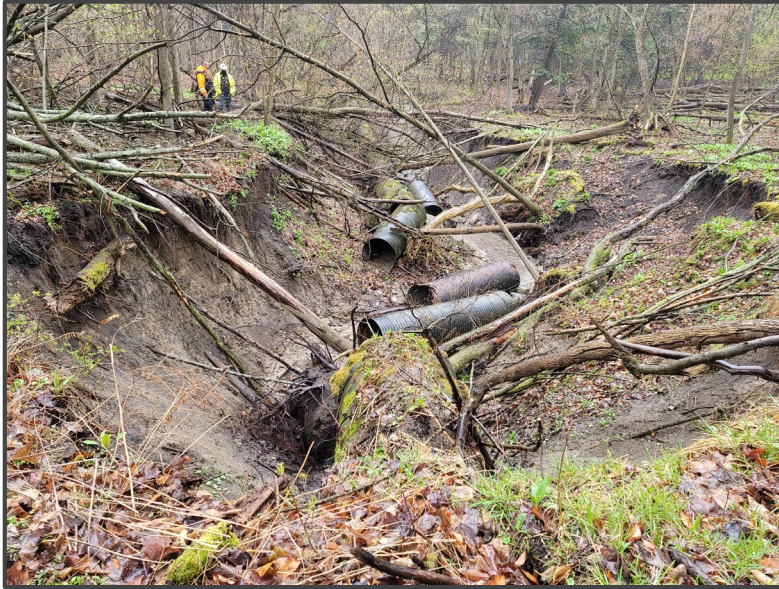
Erosion Gully Formation Along Stormwater Outfall
