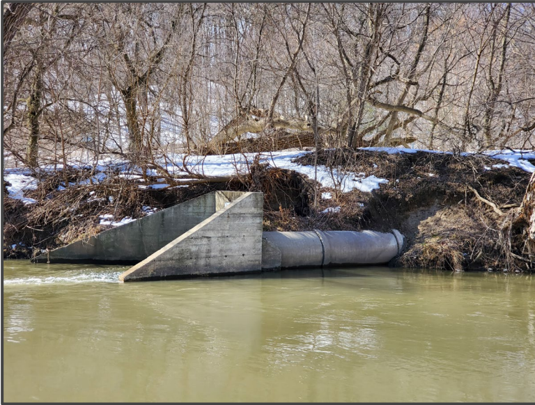
Outflanked Concrete Headwall Structure and Upstream Pipe
