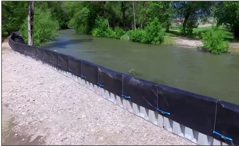
Example of Successful Field Deployment
